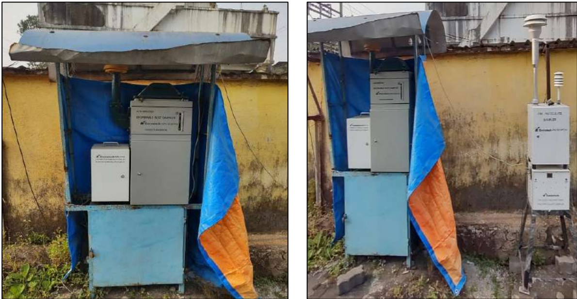
Figure 4.1: Air Monitoring System installed by PMC
